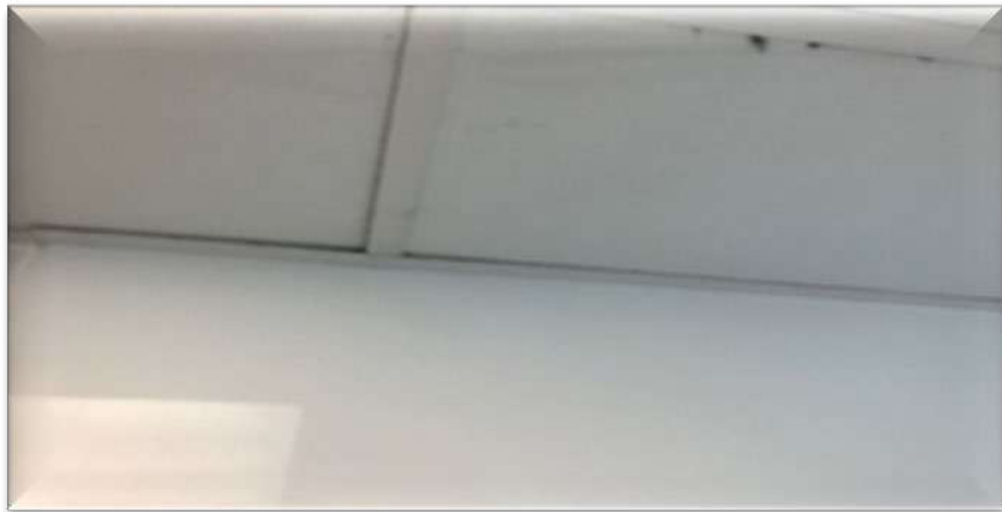
Fungal chandeliers from ceiling tiles in uncontrolled corridor
