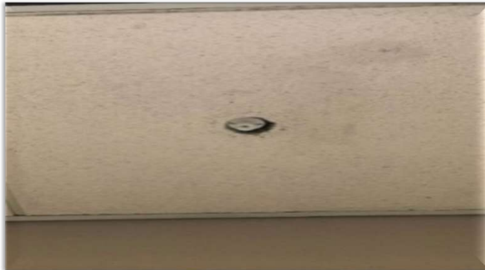
Compromised ceiling tiles and signs of leaks
