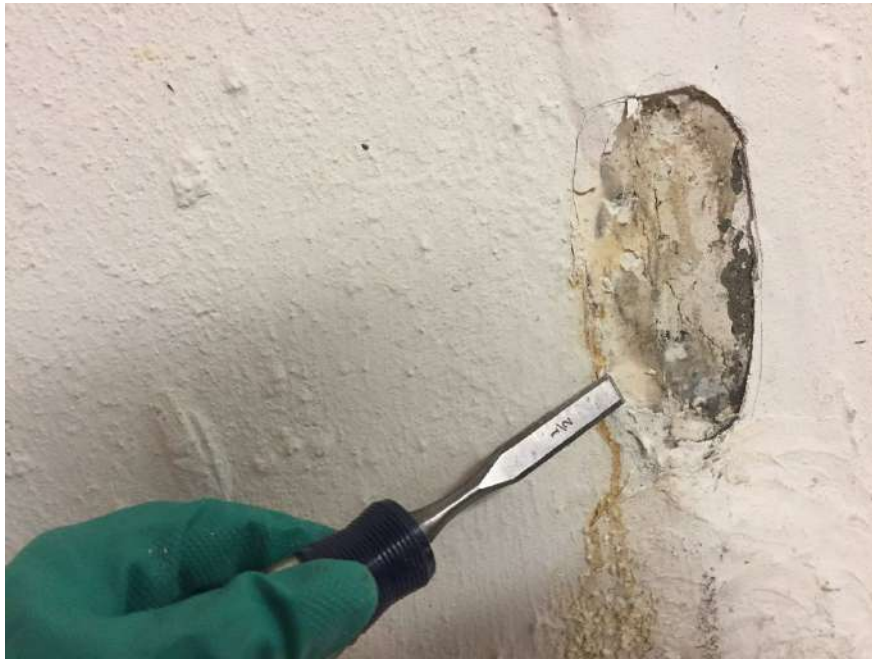
Leak in wall
